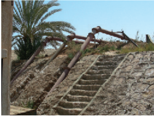
(25) Discharge pipes to a drainage reservoir (near Rashda)
