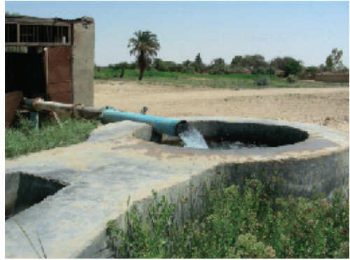
(14) Flow from an electric submerged pump
