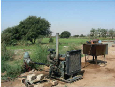
(1) Diesel-powered pump installed of water to the originally artesian well
