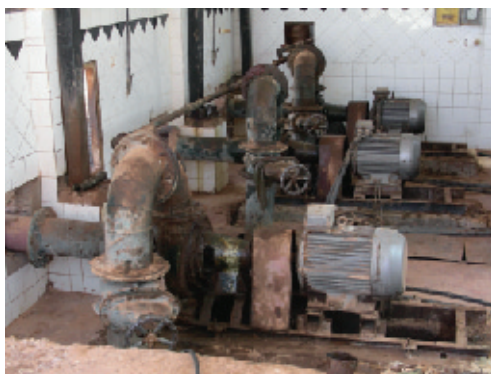
(24) Drainage pumps (near Rashda)
