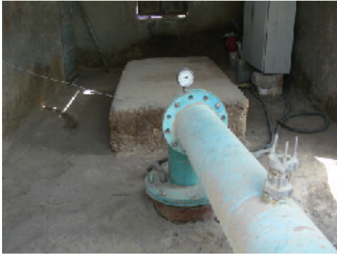
(13) Electric submerged pump
